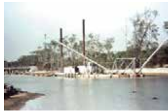
Looking across the canal with the Lake View Dr bridge in the background (1997)
