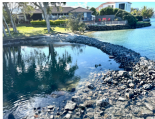
Erosion damage to the channel before repairs Barge on the channel making repairs New rock wall at end of channel
